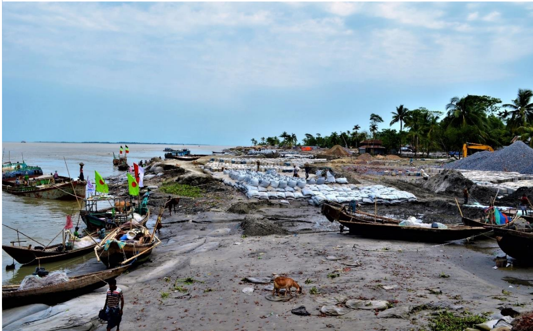
River shoreline protection works in Bhola Island, Bangladesh
